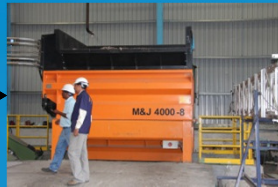
Conveyed to Primary Shredder to improve flowability
